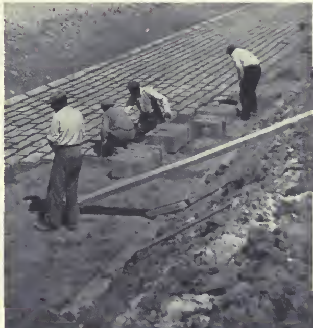
PRECAST CANAL LINING BLOCKS are set in the irrigation canal on Brian project in the Veneto region of Northern Italy.
